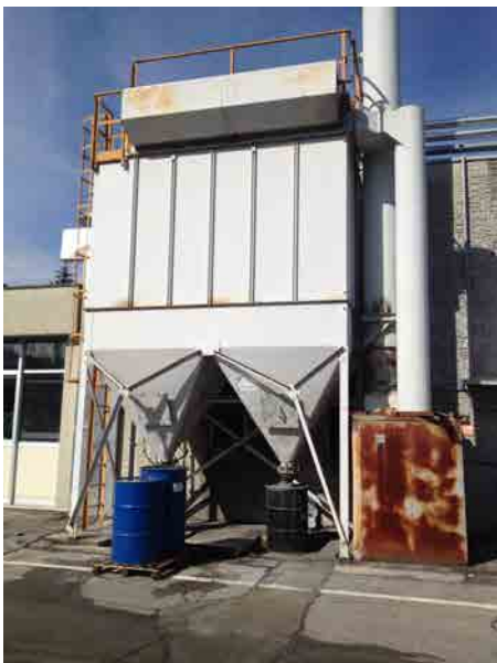
Impianto obsoleto. Obsolete plant (to be disassembled)
